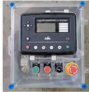
DG ENGINE CONTROL PANEL
