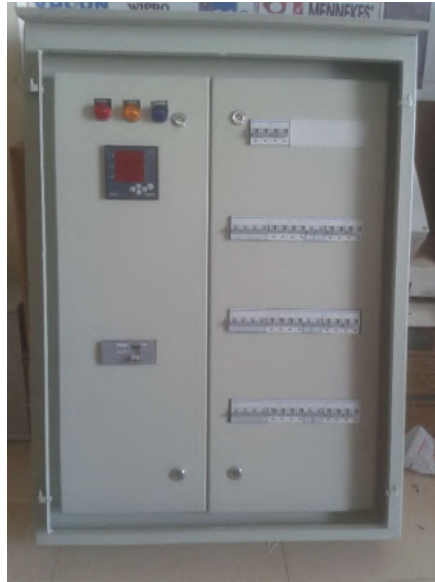
MCB Distribution Board
