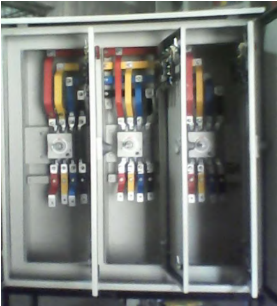
Feeder Pillar Panel
