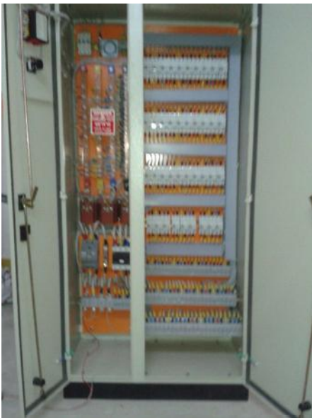
Lighting Distribution Board
