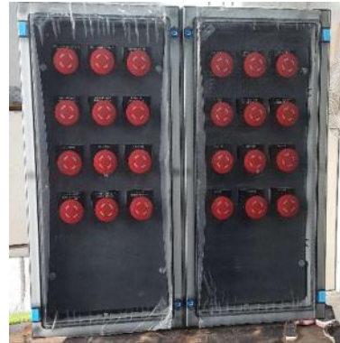
LOCAL CONTROL STATION
