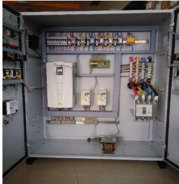
VFD Control Panel
