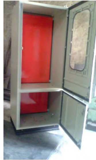
UPS / BATTER BOX
